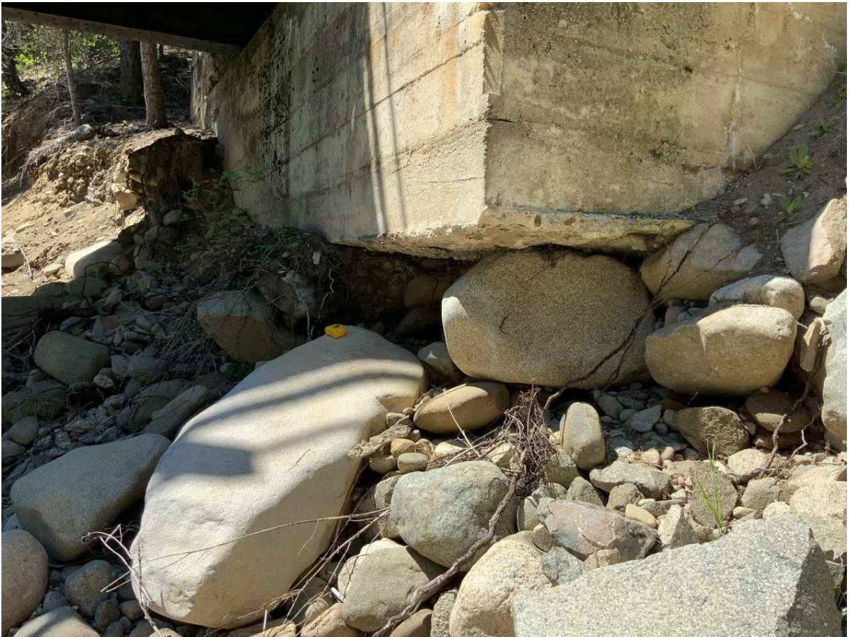
PHOTO 4: UNDERMINING AT THE "RIGHT" ABUTMENT
